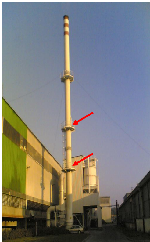
Figure 1: Exhaust with measuring point AM2
